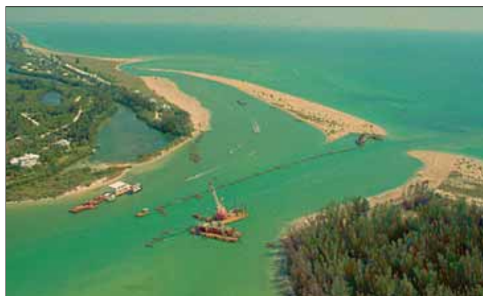
In April 2003 this was the state of the alignment dredging. Before the dredging, boats had to make their way down the sandsprits and through the curved and changing shallows.
