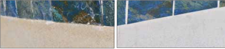
Before and after the acid wash. The pool walls went from yellow to blue white
